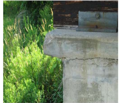
Close up of Damaged Concrete Cap (Northeast Side)
